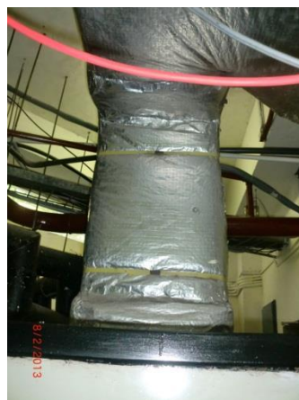
AHU MAIN DUCT
