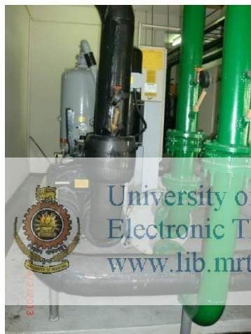
CHILLED WATER PIPING
