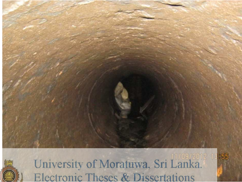
Figure (a): Corroded penstock (Original in colour)
