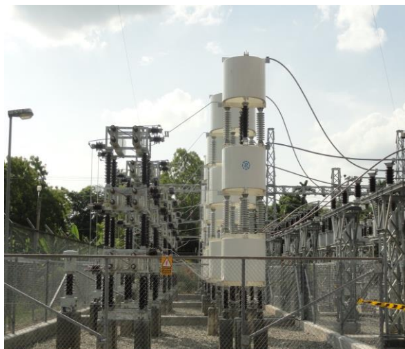
Figure 2.11: Stacked rack mounted
