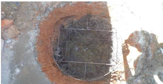
Figure 48: Earth mesh In Pole Pit
