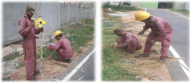
Figure 14: Earth resistance Measurement at Field
