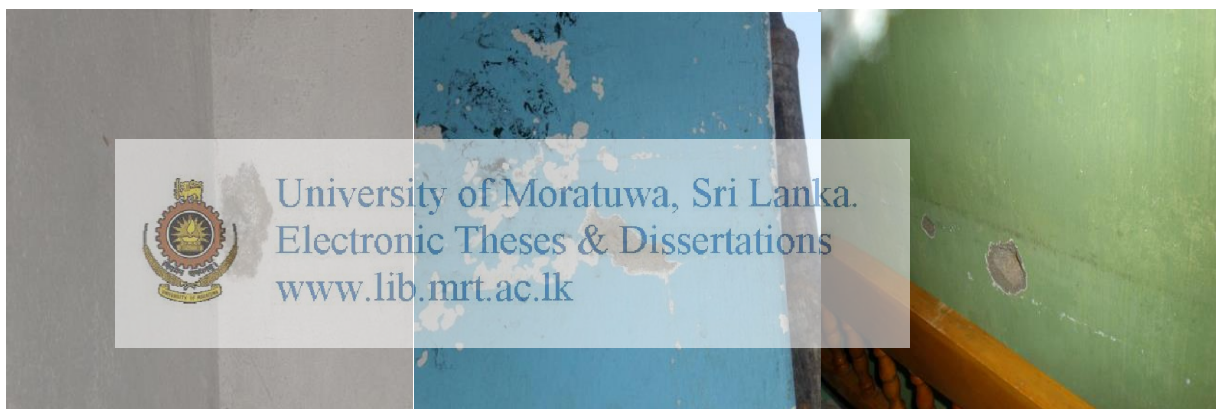
Figure 3.21: wall damages reported in homes near the Nakiyadeniya telecommunication tower
