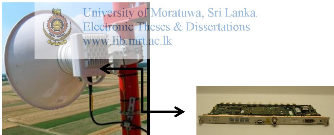
Figure 3.13: MW Outdoor and Indoor units connected through IF cable (Source: Author)
