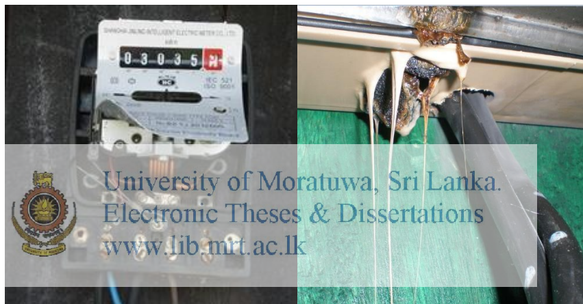
Figure 3.18: Energy meter and cable damages reported near the Keselhenawa telecommunication tower (Source: Author)
