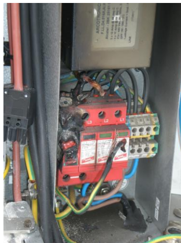
Figure 3.19: Neutral to earth surge arrester damaged in Magalle radio base station (Source: Author )
