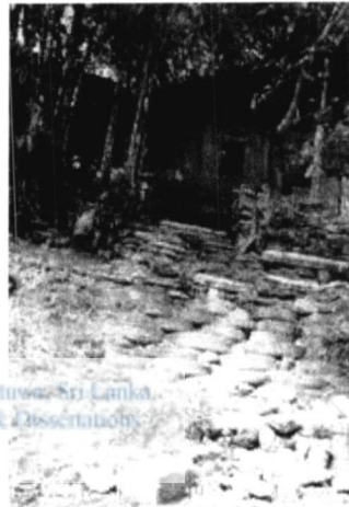
Figure 36: Retaining wall River edge retaining wall made from discarded tires filled with garbage.
