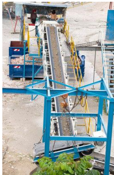
Figure 2. 5: Construction Waste Recovery Facilities Placed in Sarimbun Recycling Park
