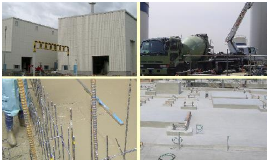
Figure 2. 8: Project No.2; Incinerator Building Installed in the Yokohama Thermal Power Plant Premises
