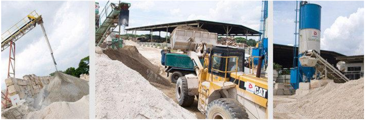
Figure 2. 4: Construction Waste Recovery Facilities Placed in Sarimbun Recycling Park
