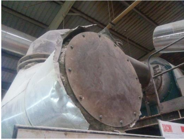
Figure 7-1: Weak thermal insulations
