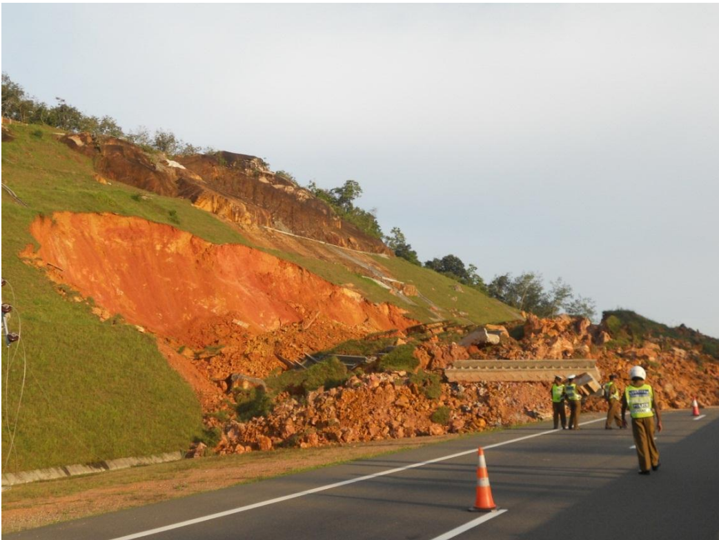
Figure 3.11 – Debris of Failure Has Covered the road section towards the Galle
