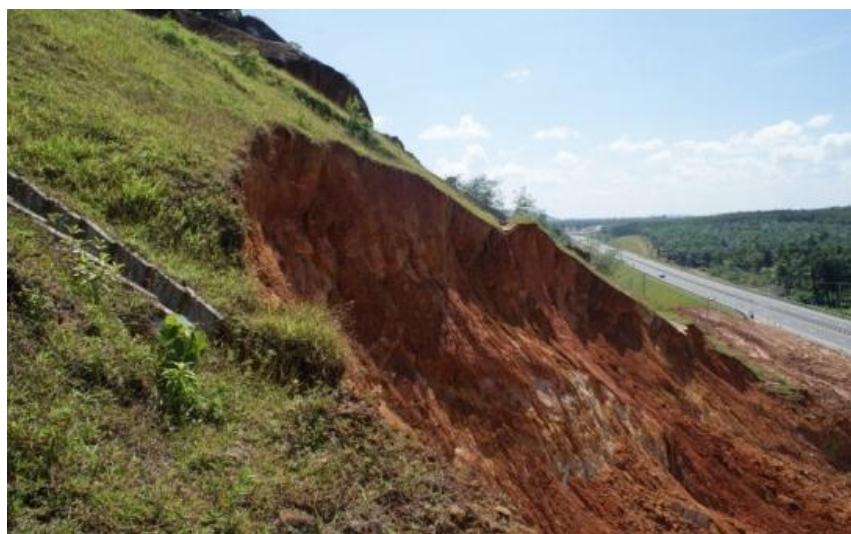
Figure 3.12 –A Zone of whitish Feldspar rich clay in the failure surface
