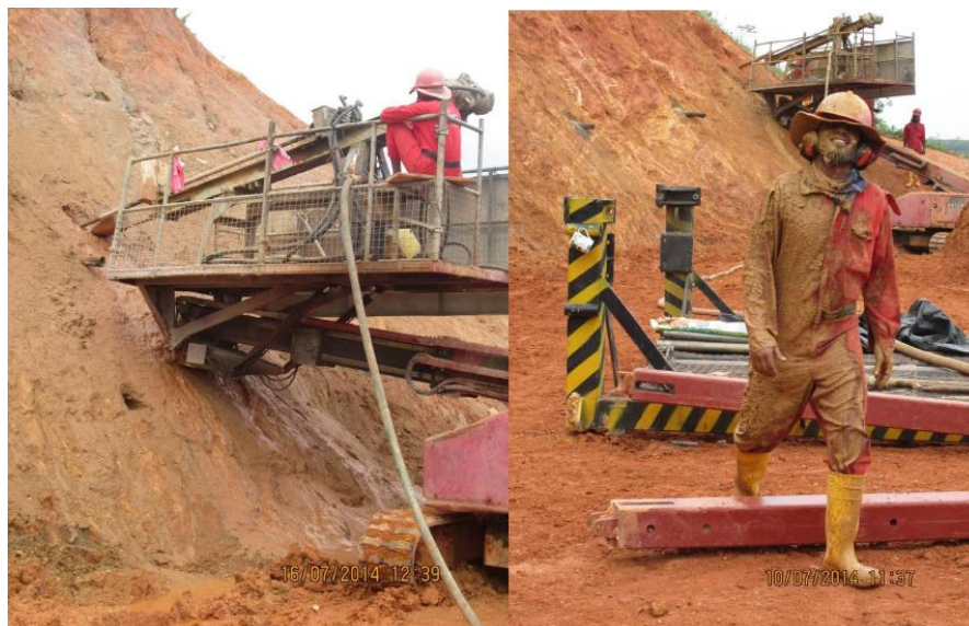
Figure 3.4 – Water oozing out of relict joints during drilling
