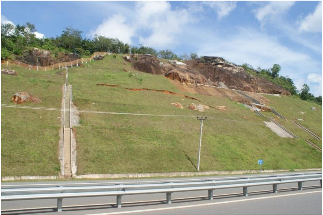
Figure 3.8 – Initial Crack and downward movement of soil
