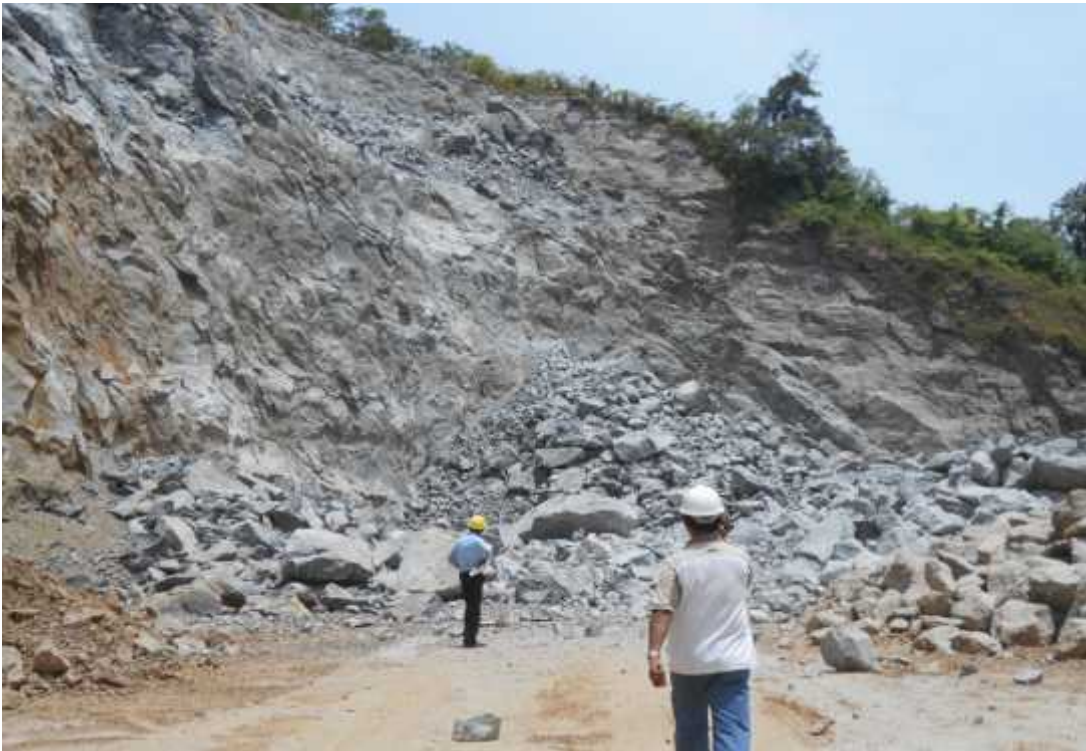
Figure 7.36: After the blast the rocks which fell below in phase 10
