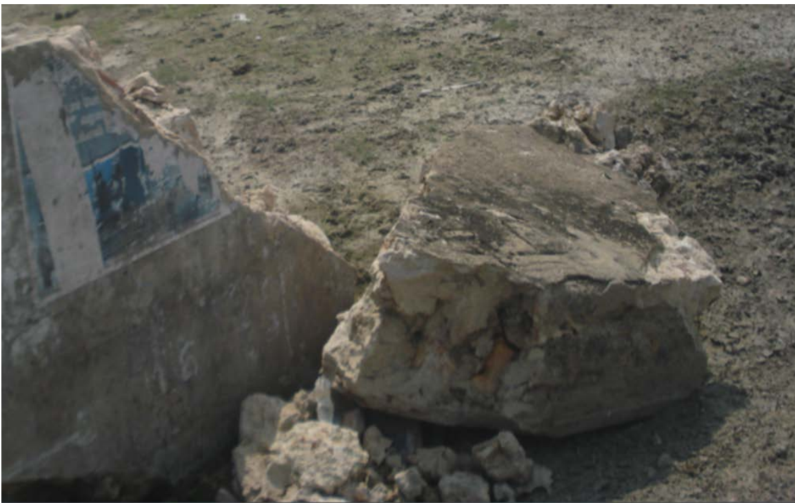
Figure A15.2: Concrete Debris
