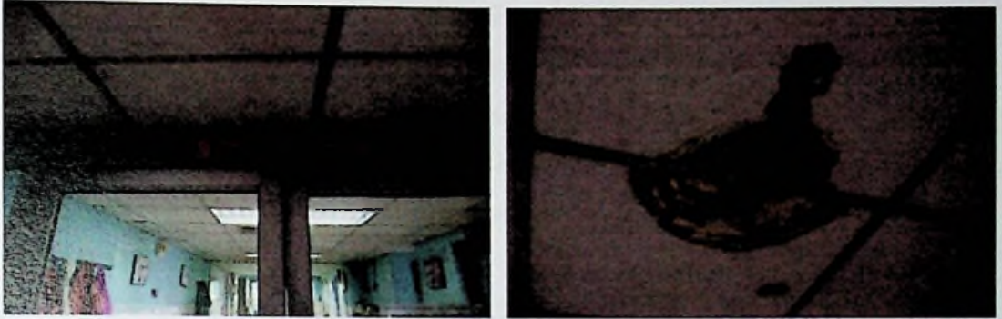
Figure 3.6: Ceiling affected due to condensation
