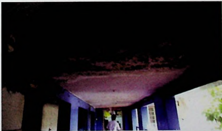
Figure 3.4: Improper rectification work to corroded slab reinforcement
