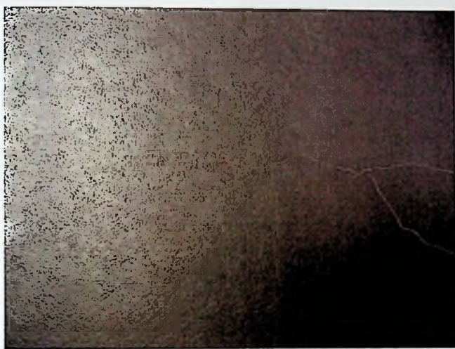
Figure 3.11: cracks in Eye Unit LRH
