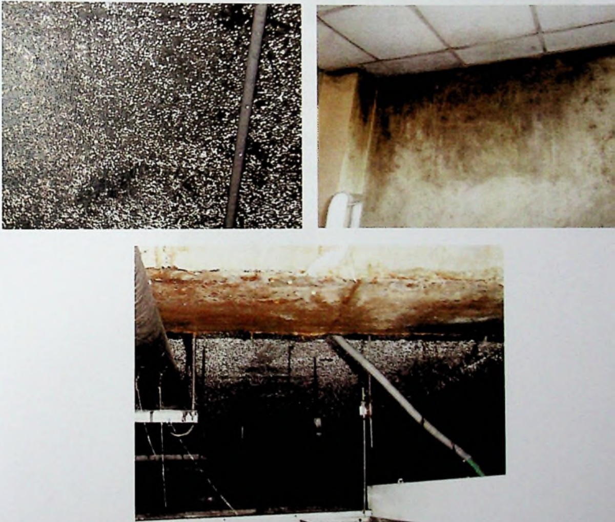
Figure 3. 5: Condensation and accumulation of water under slab soffits at NINDT
