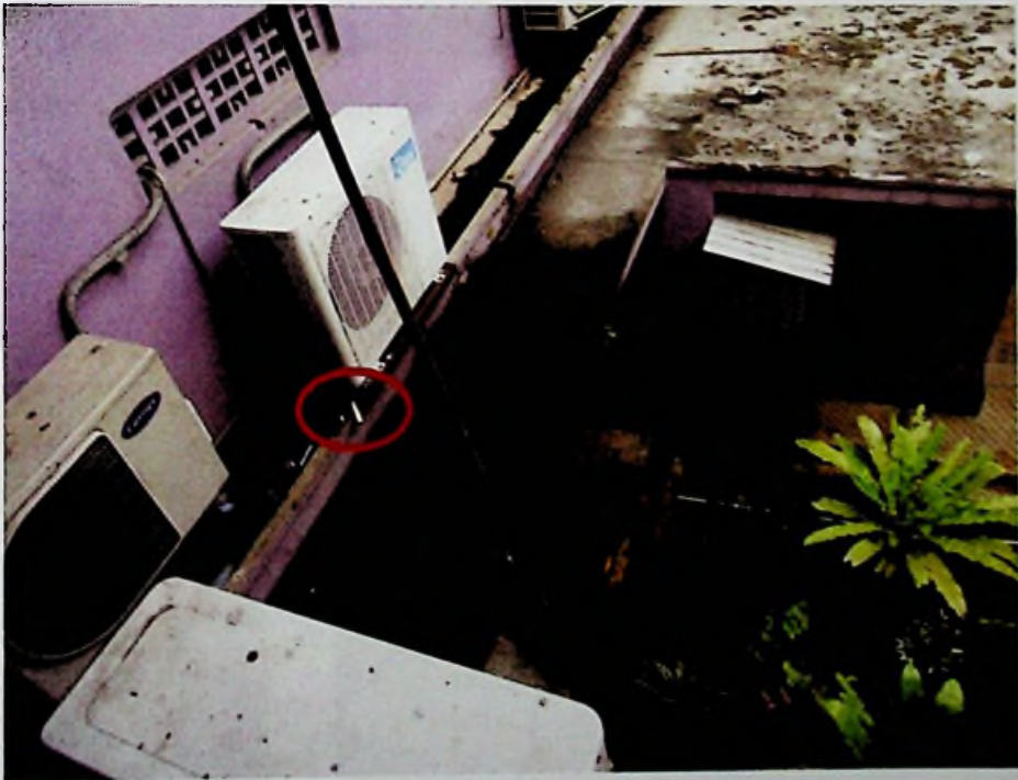
Figure 3.17: Improper arrangement of A/C Outdoor units
