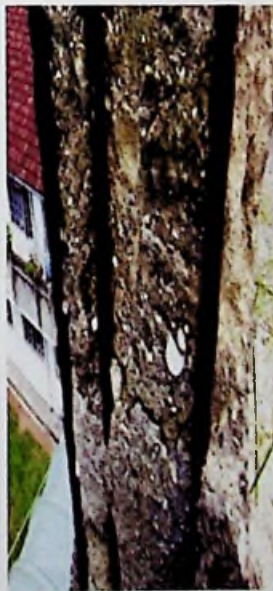
Fig 3.7: Severe corrosion of reinforcement of column concreted using sea sand at NCTH - Ragama
