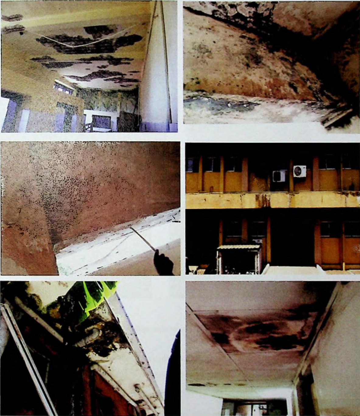
Figure 1.2: Deteriorated situation of GHBs
