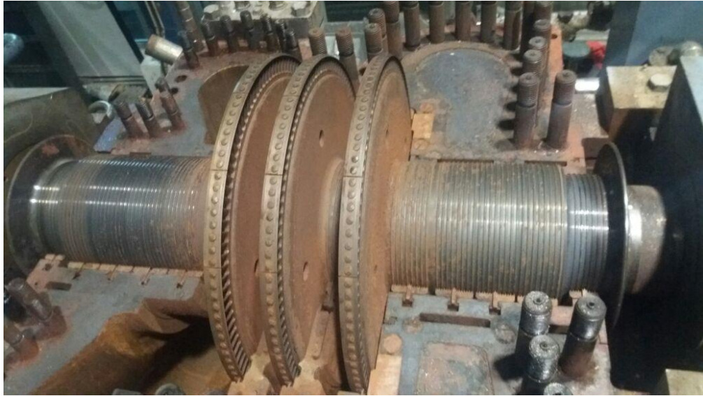
Figure 17: Steam turbine upper half opened for inspection
