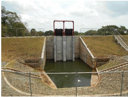
Figure A.7: LB Sluice (New) (LB Low Level Sluice) (original in colour)
