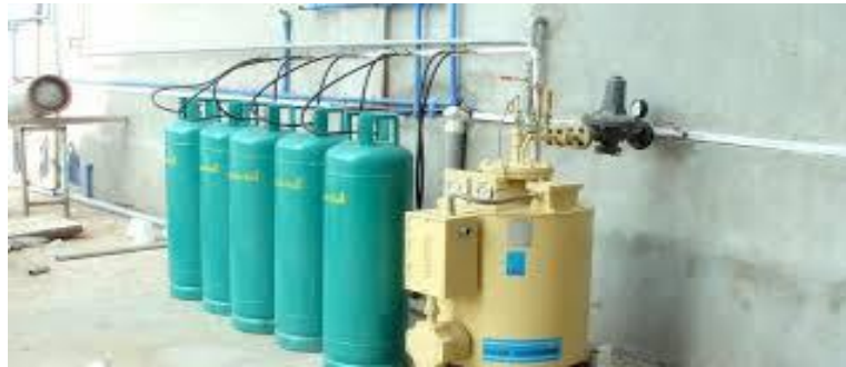
Figure 17: Liquid withdrawal manifold with Vaporizer
