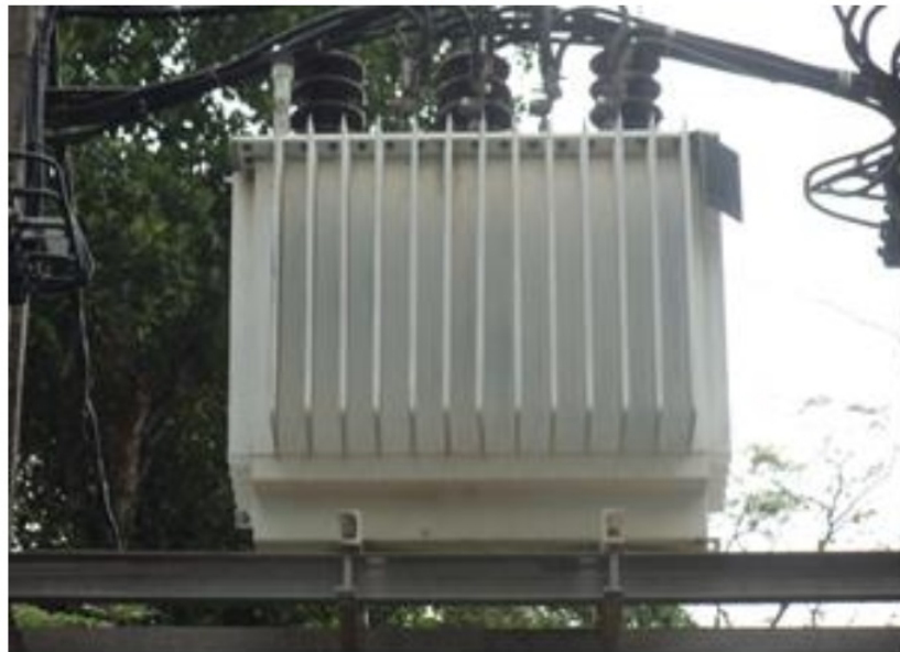
Figure 1.7: Coconut oil filled 160 kVA, 33/0.4 kV distribution transformer installed at Wathara, Kesbewa, Sri Lanka [31].
