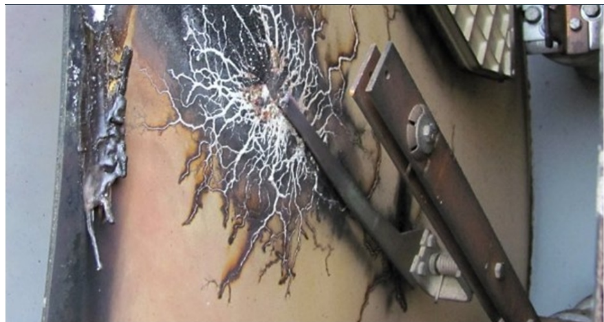
Figure 1.6: Discharge formation in a distribution switchgear [29]
