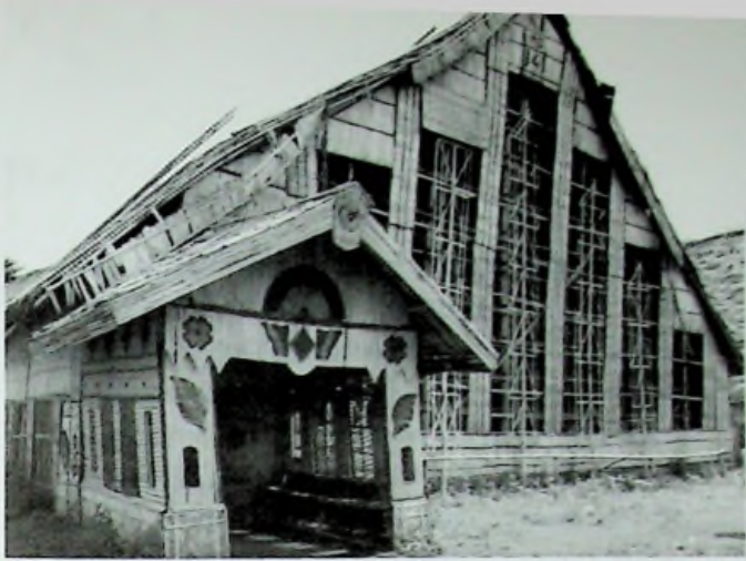
Figure 11: Jember's Los damaged by harsh wind. Source: Author's documentation, 2010
