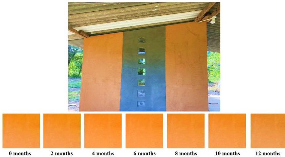
Figure 7.35: Colour variation of sludge putty applied on exterior wall with shade
