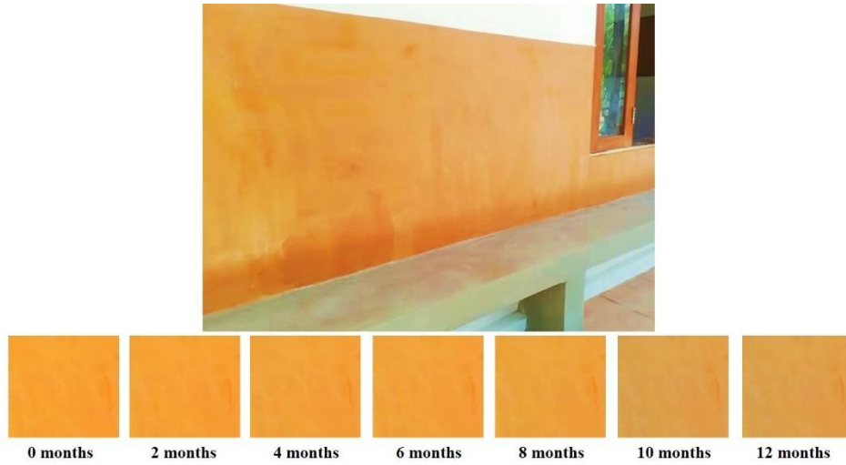
Figure 7.34: Colour variation of sludge putty applied on exterior wall
