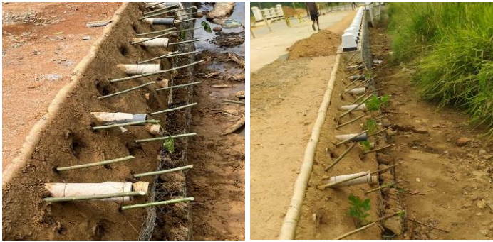
Figure 14 Photographs taken at Location 2 on 21.03.2024 after the stabilization technique
