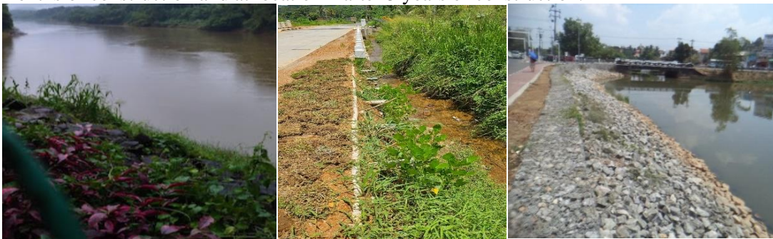
Figure 22. Photographs taken at Location 1, 2 and 4 showing the post-construction performance of the adopted stabilization techniques
