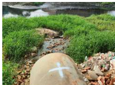
Figure 10: Sewerage line opens at canal front.
