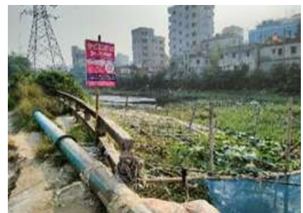
Figure 11: canal-side broken walkway
