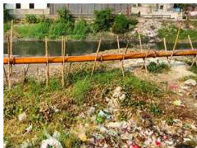
Figure 13: Sand carrying pipe over canal.
