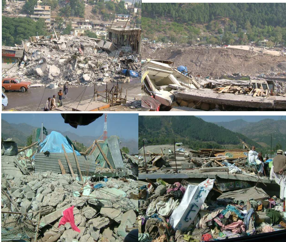
Figure 2: Structural damages due earthquake
